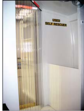
Airlock Clear Strips & SCSR Disposal bin
