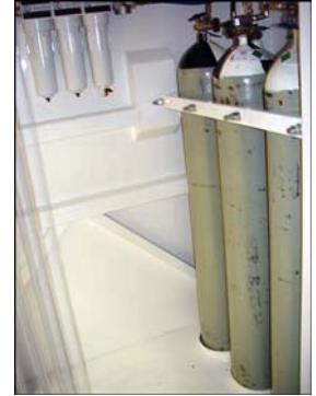
Oxygen cylinders & filtration system
