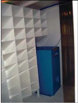
SCSR Storage Racks & CO 2 Scrubber
