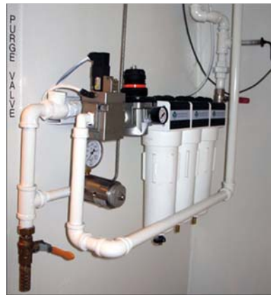
Mine Air Filtration System
