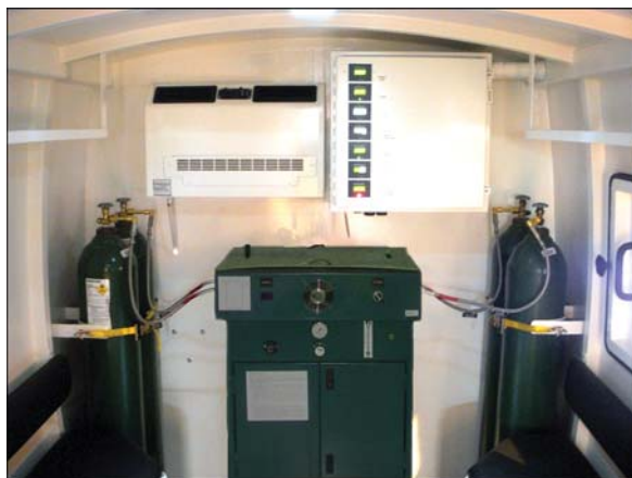
Scrubber, air conditioner and chamber monitoring system
